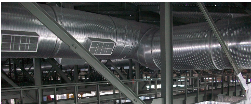
Quality Mechanical's ductwork at the T-Mobile Arena in Las Vegas.
