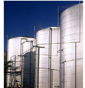
Lignotech External Tanks, Mt. Vernon, WA
