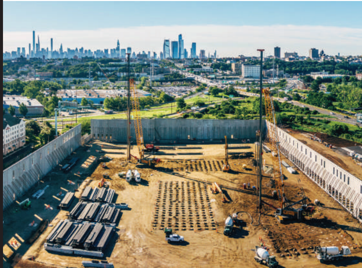
As part of the Lincoln Gateway project, Menard Group USA ( No. 166 ) installed rigid inclusions to depths of up to 175 ft to support a 326,000-sq-ft distribution center in Secaucus, N.J., the firm says.
